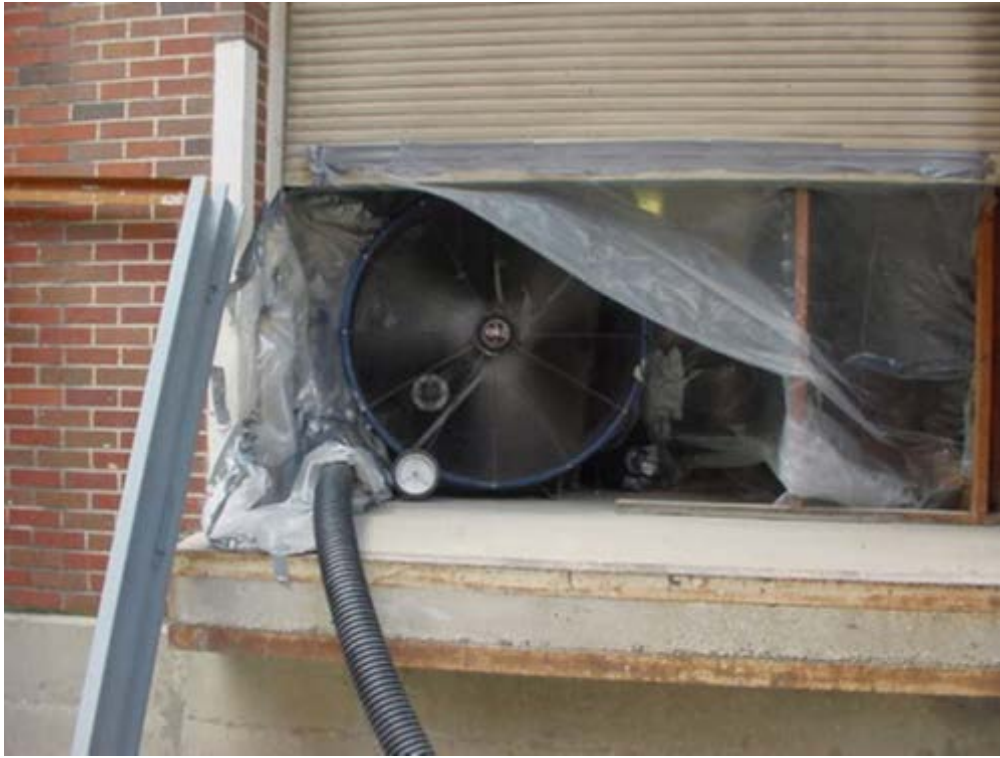
Photograph 9-6 View of ventilation with an industrial fan
