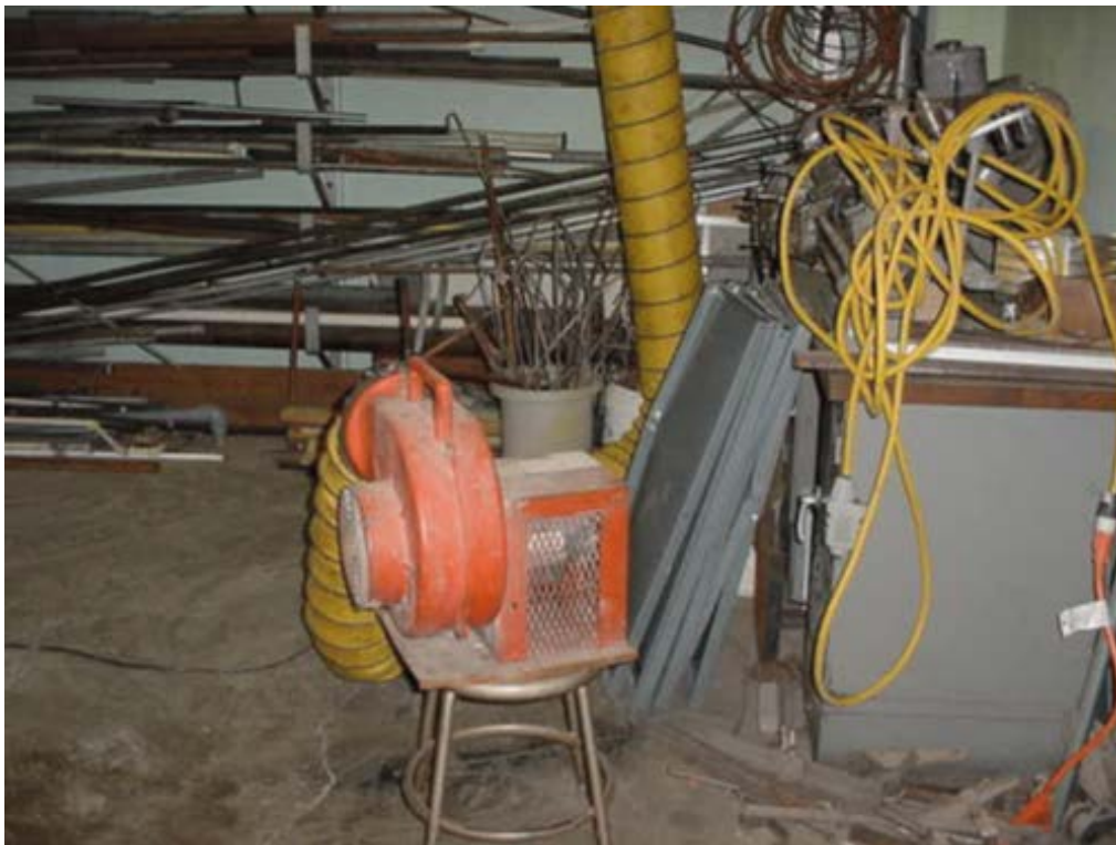
Photograph 9-7 View of ventilation with a blower unit
