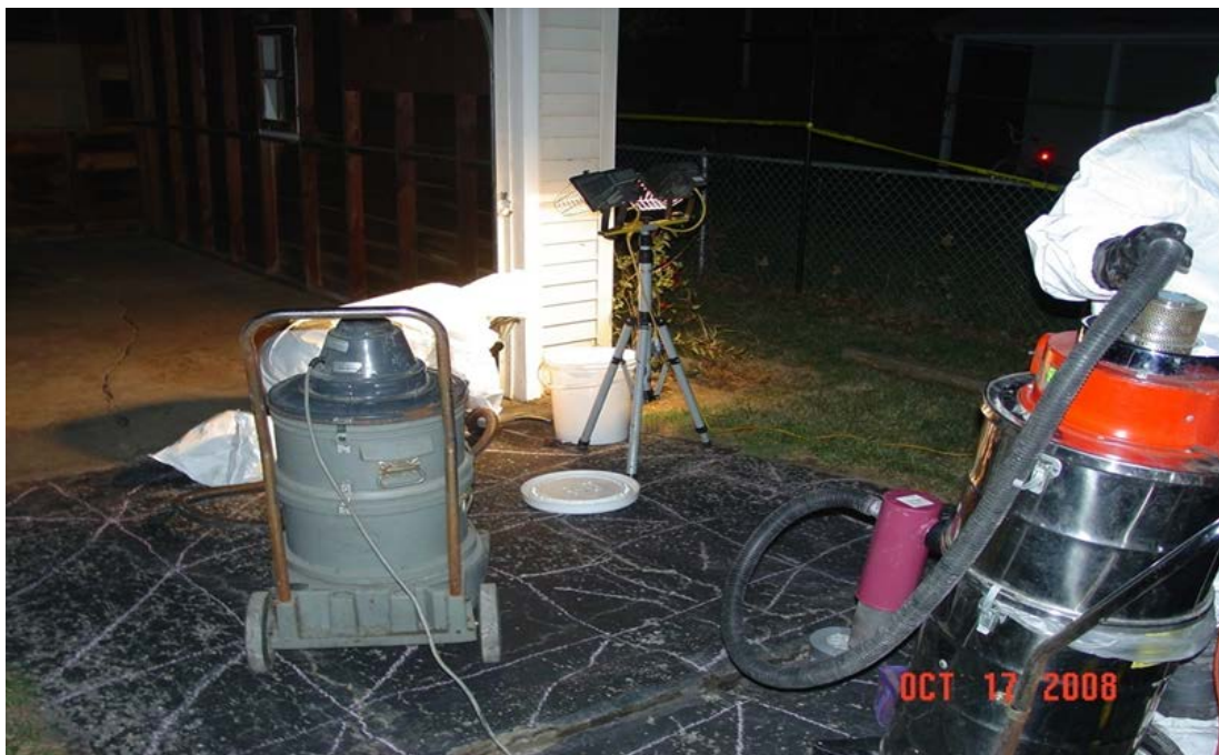
Photograph 9-20 View of grid system marked on asphalt where mercury vacuuming has been completed
