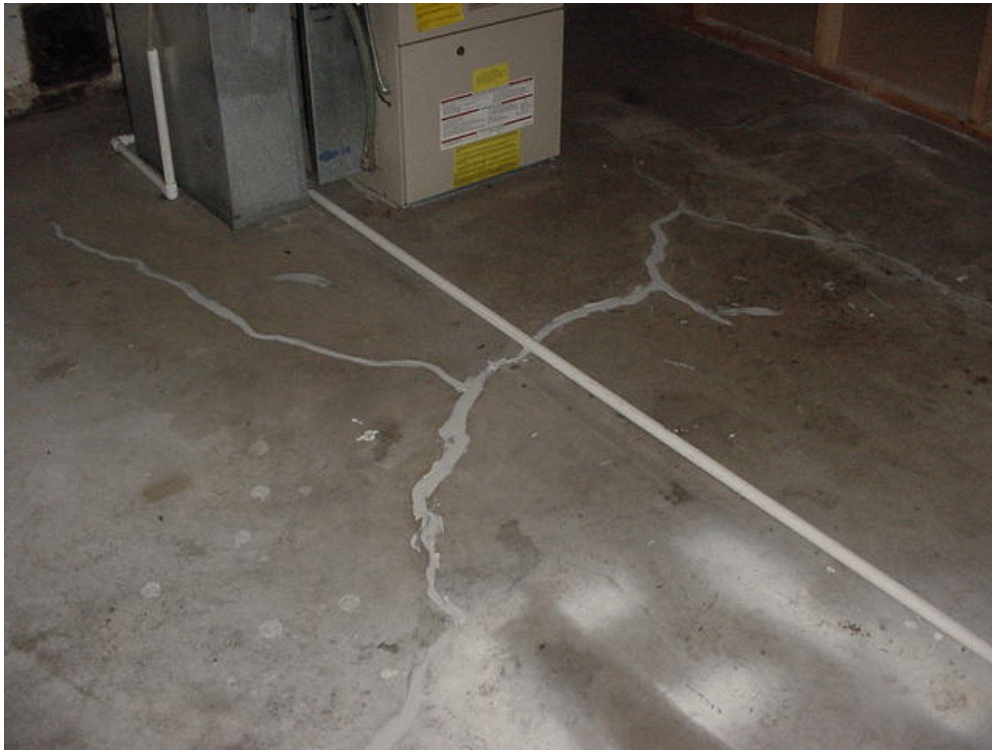
Photograph 9-8 View of floor cracks sealed with caulking material
