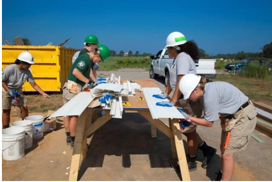
National service members of AmeriCorps NCCC (National Civilian Community Corps) work in sweltering (100°F) Alabama heat to help rebuild homes destroyed by a tornado. (Photo credit: Christopher Mardorf, FEMA)
