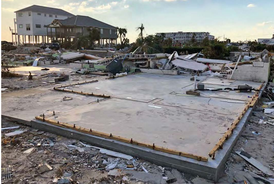
Figure 3. Remaining slab of a non-elevated structure from Hurricane Michael
