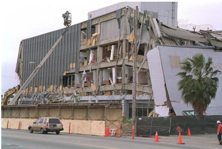
Figure 4. Damage from Northridge Earthquake
