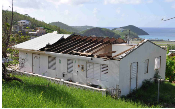
Figure 2. USVI home built using pre-1994 code
